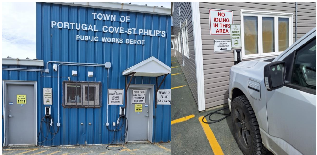
Figure 2.3 EV Chargers at Town Depot and Office
