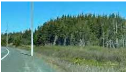
Existing pole line
