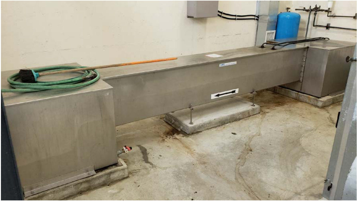
Photo 1: Side view of existing UV unit.
