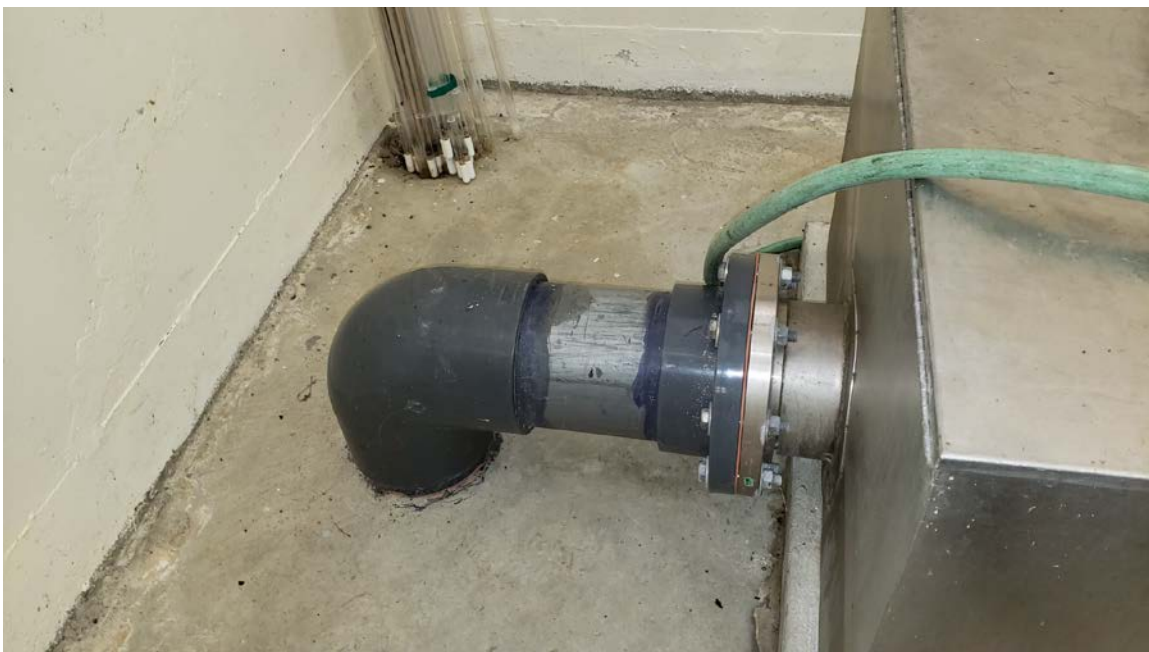
Photo 4: View at outlet from existing UV unit.
