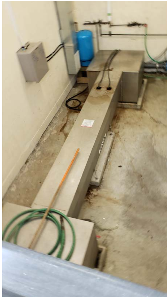
Photo 2: Top view of existing UV unit.
