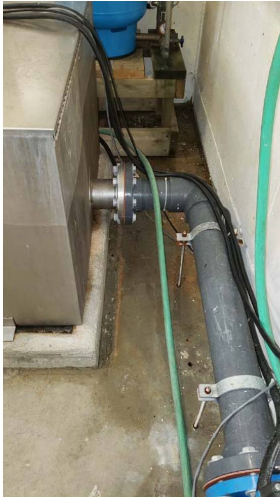
Photo 3: View at inlet to existing UV unit.
